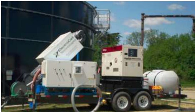
Figure B- 9. representative installation Bio-Electric technology
