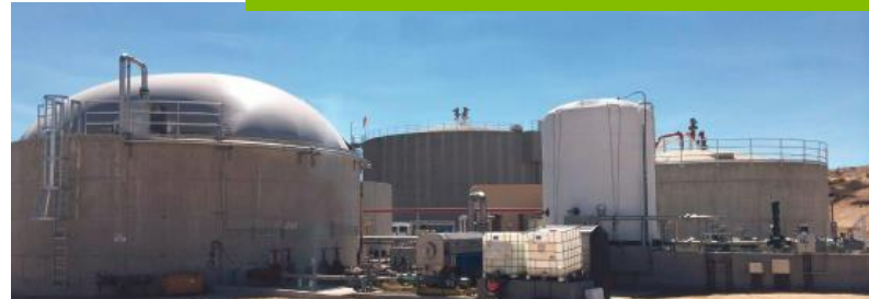
Victor Valley, CA, Digester converted into an Omnivore™
