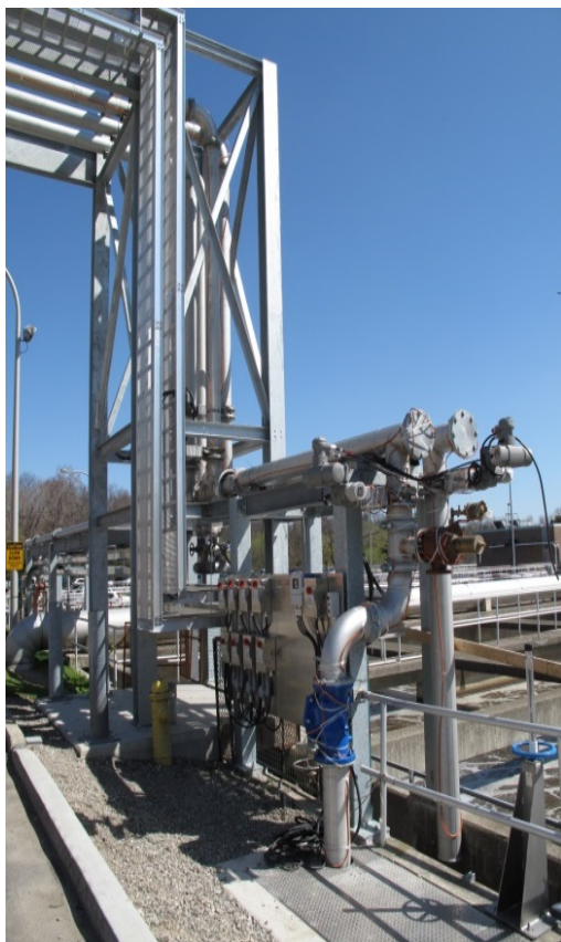
Unique supply infrastructure associated with OWC's London Wastewater Facility
